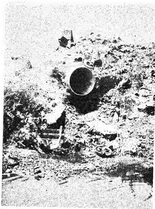
Figure 20. Upper end of a highway culvert placed too high for drainage. This results in mosquito breeding pools upstream from the culvert
